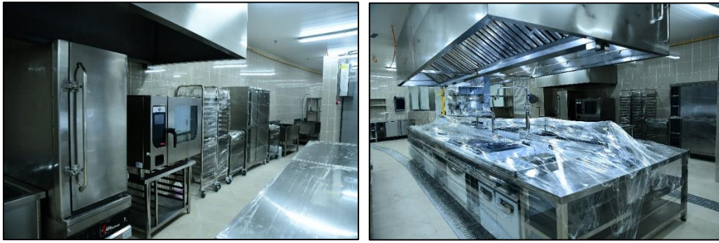
Figure 31: Lotus Tower - Kitchen
